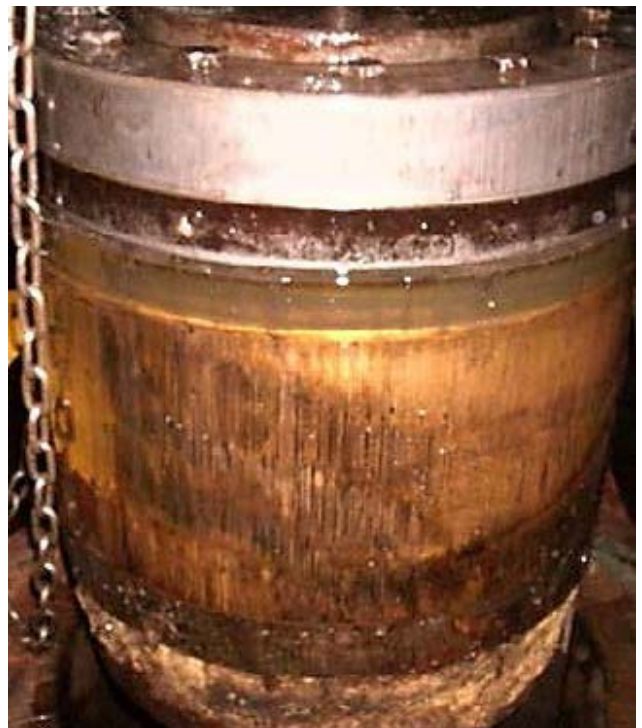
Shrunk piston seal and severely scratched/worn-out bronze surface of ram
